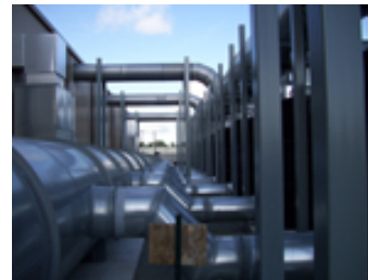
The 90-inch diameter duct on the exhaust side leading from charcoal canisters.
