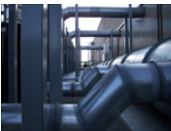
Close up of ductwork and 12x12x3/8-galvanized
