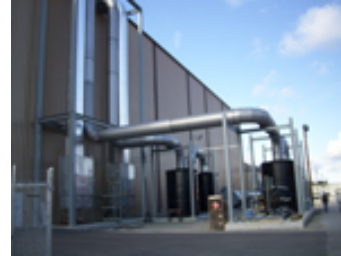
Duct from charcoal canisters to the 70-foot elevation into the facility's Building A.
