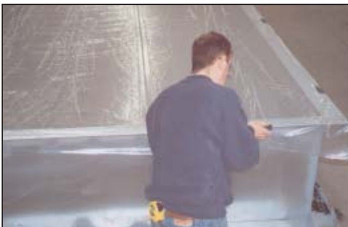
Limbach craftsman Scott Sneddon seals a piece of cleaned, fabricated duct using swimming pool clips.
