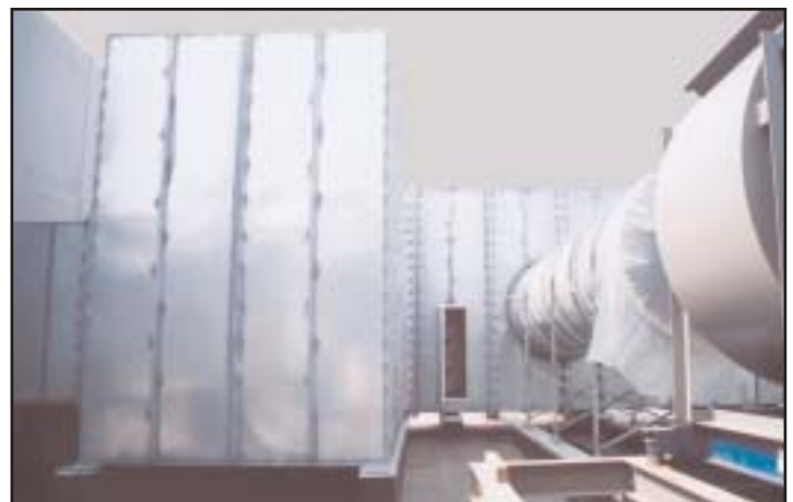
The completed lab/office roof exhaust plenum with the fans tied in after assembly.
