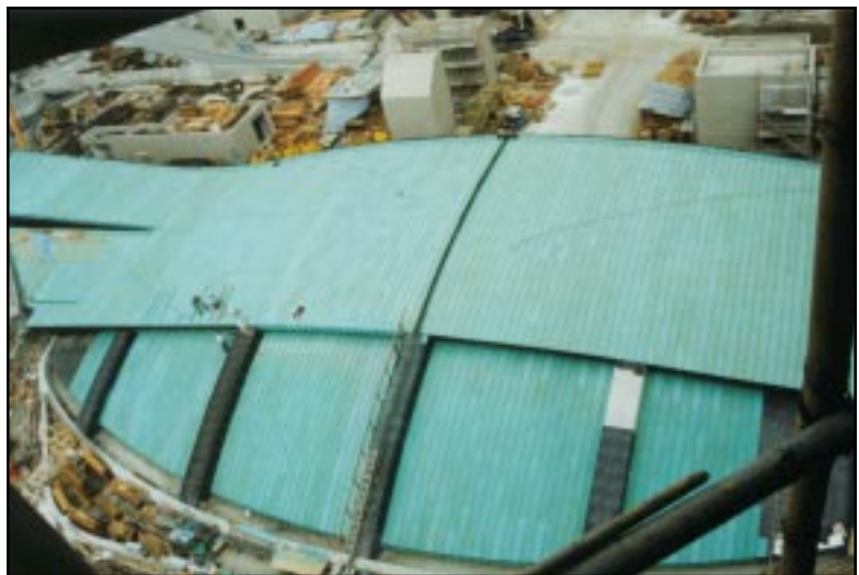
Pre-patinated copper installation by A. Zahner Company of Kansas City, Mo. The Tsing Yi Mass Transit Station is the largest copper roof installation in China.
