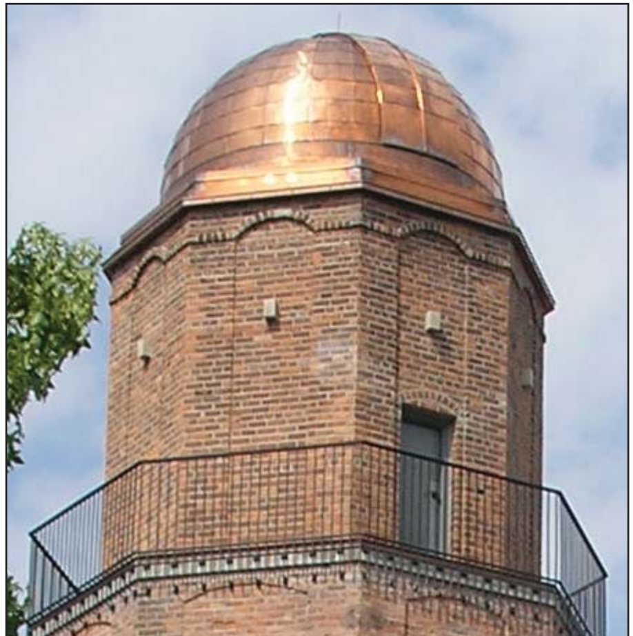
The polished Cranbrook Observatory dome was completed and installed in just two months.
