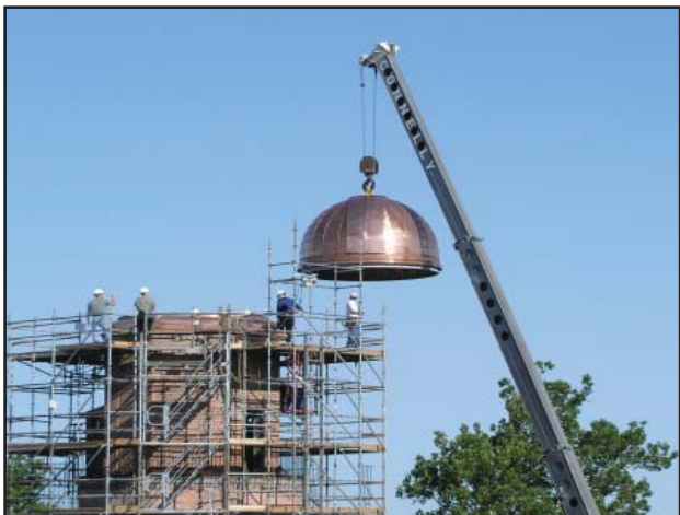
The burnished 5,800-pound dome is hoisted 80-feet high to its new home.
