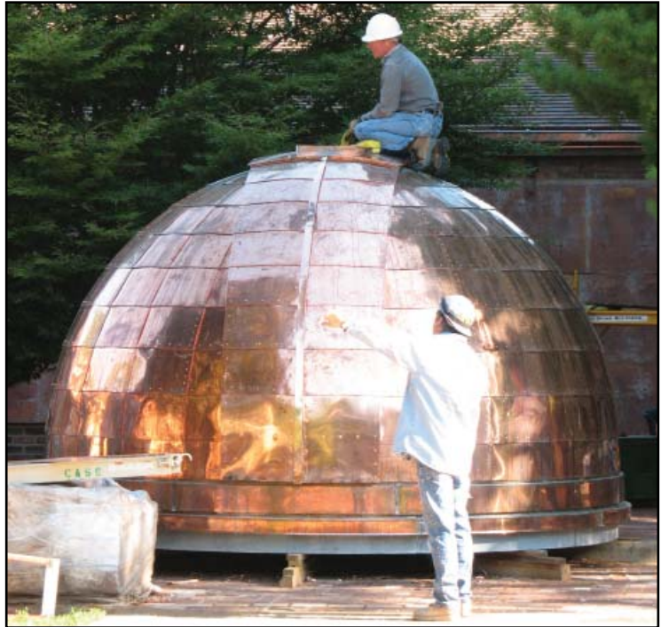
C.A.S.S. employees prepare to hoist the shimmering new dome to its new home atop the Cranbrook Observatory tower. C.A.S.S. preserved the dome’s historic intent by emulating the original rivet pattern without penetrating the panels. All seams were soldered watertight.
