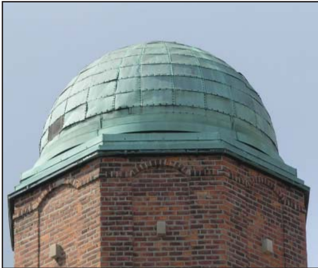
Wind and water damage had taken their toll on the original Cranbrook Observatory dome.
