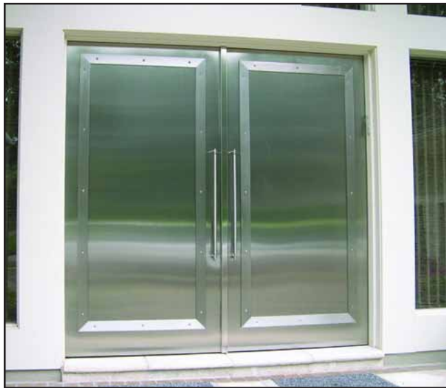
A 16 gage #3 stainless steel sheet was used to clad over the existing doors with a 38 inch by 3 inch stainless steel brush finished flat bar.
