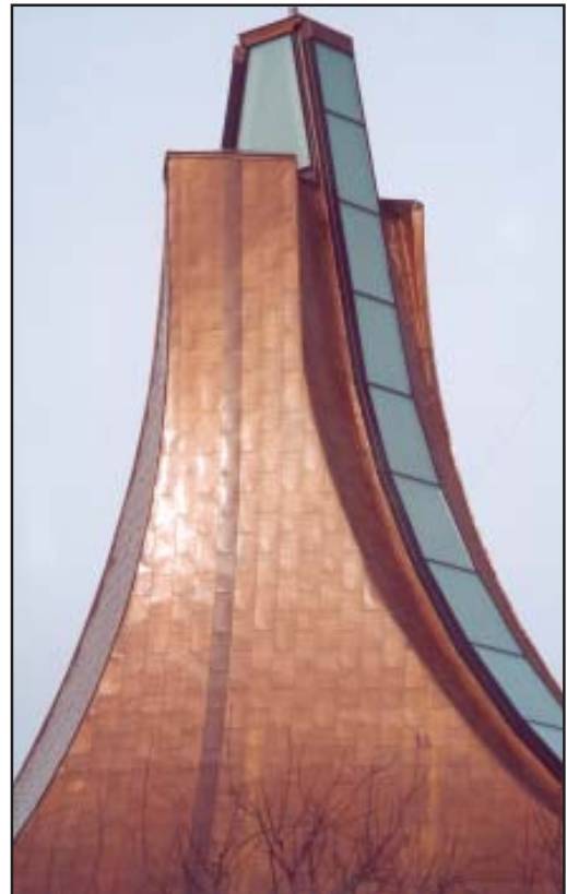
Even to an untrained eye, the importance of the sequencing and layout of the copper panels on this project is easily apparent. The 16-ounce flat-lock copper panels are perfectly aligned from roofline to peak.
