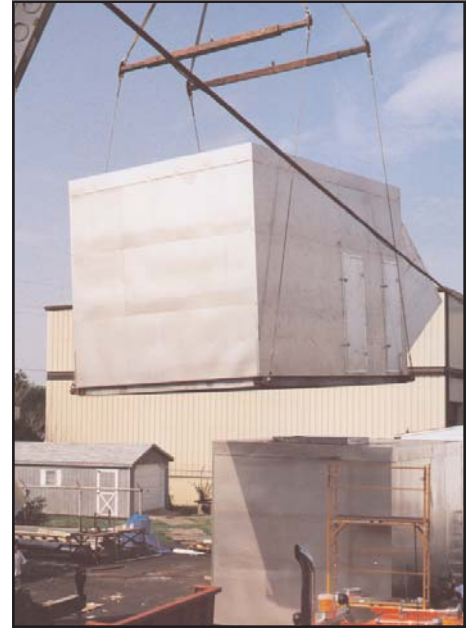
Each completed unit was installed on the roof of the five-story facility.
