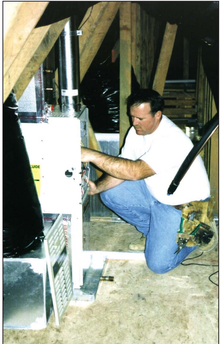
Working within a confined attic, Tom Heise, journeyman, is performing a furnace installation.
