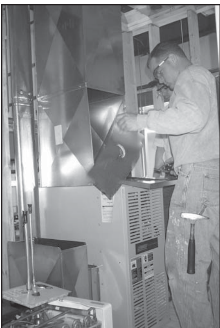
An apprentice is installing a furnace supply plenum on one of the 10 systems used for residential installation work training.
