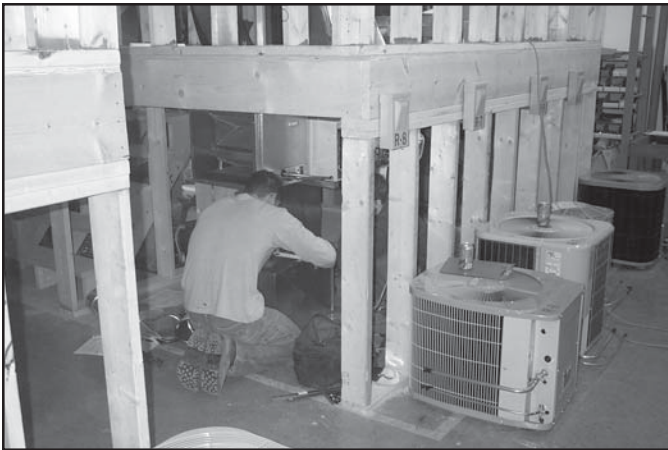
This apprentice is installing a supply plenum on a horizontal gas furnace in the crawl space mock-up. The apprentices are broken up into two-man teams that will install a complete heating and air conditioning system.
