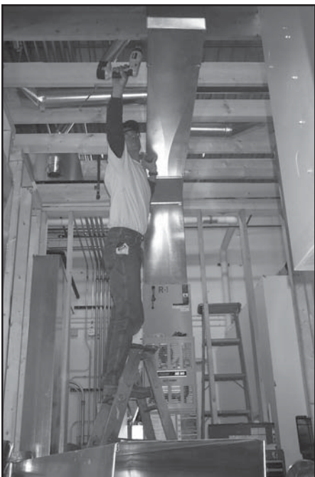
This apprentice is installing ductwork on the mock-up of a simulated basement and crawl space during training on residential installation work. Apprentices also learn sheet metal fabrication and layout, welding, AutoCAD drawing, manual J load calculation and design.
