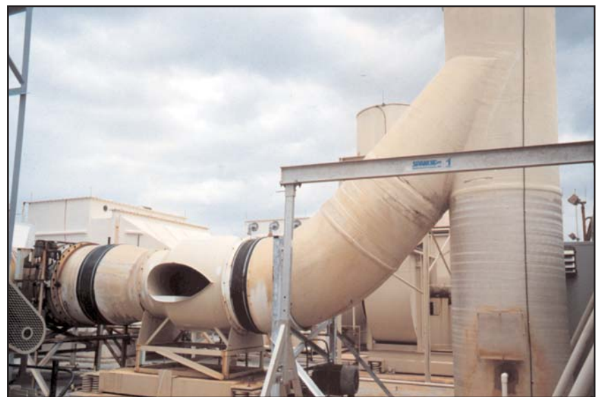
Above: The scrubber fan and stack is one of 13 that services the Arlington facility.
