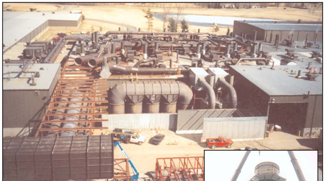
The impressive maze of 10-gage metal ductwork was installed on the exterior of Venture Industries during the cold Michigan winter.
