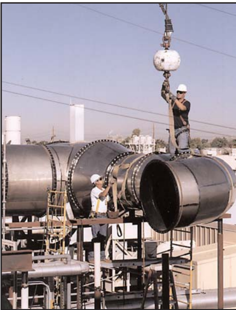
Crew members carefully installing a segment of the 1,240 linear feet of acid duct.
