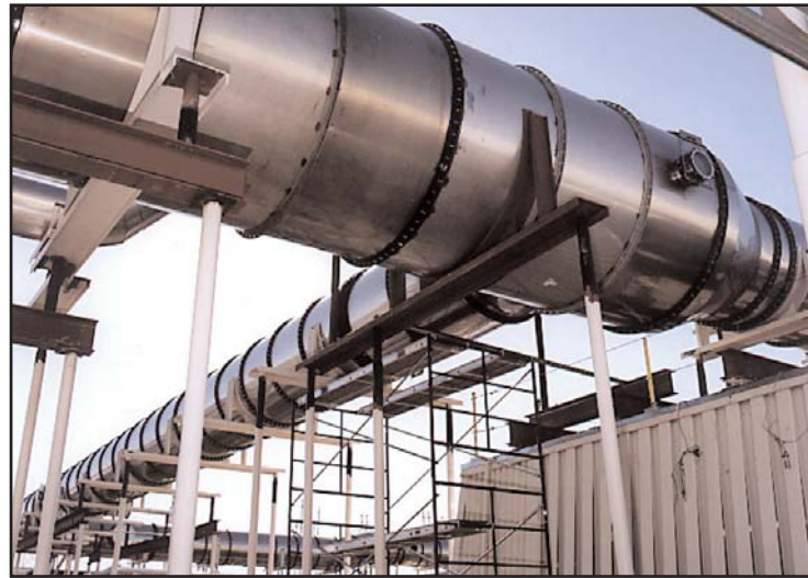
Detailed view of a portion of the Motorola plant ductwork.
