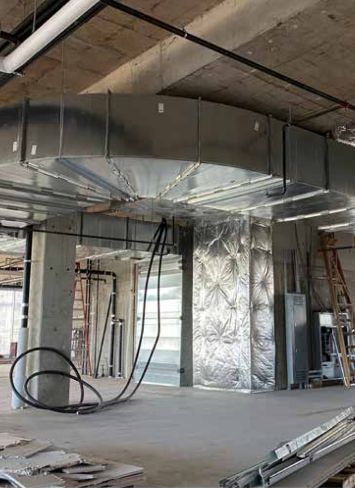
Summit Sheet Metal Ltd. installs complete HVAC systems for high- and low-rise residential buildings — all without having their own shop for fabrication. Photos: Summit Sheet Metal Ltd.
